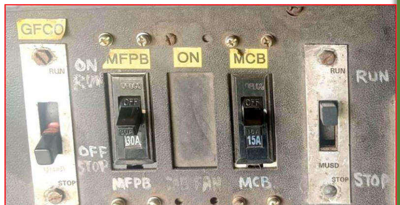
Trailing Loco MCB Position
